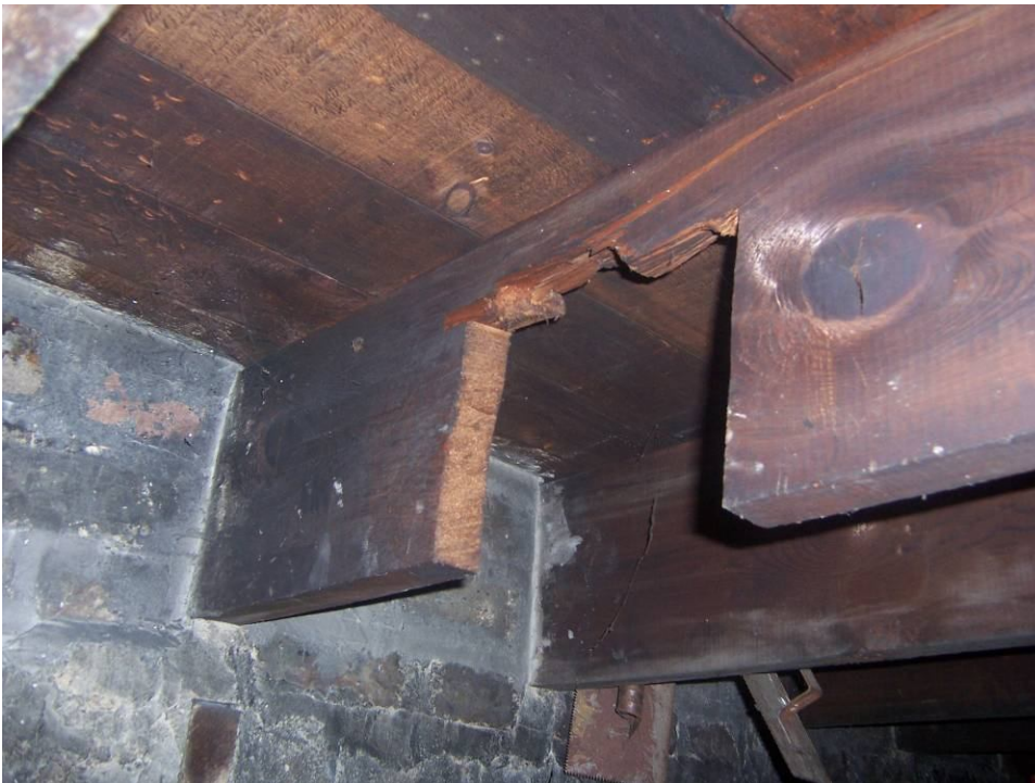
Floor joist has been notched excessively
