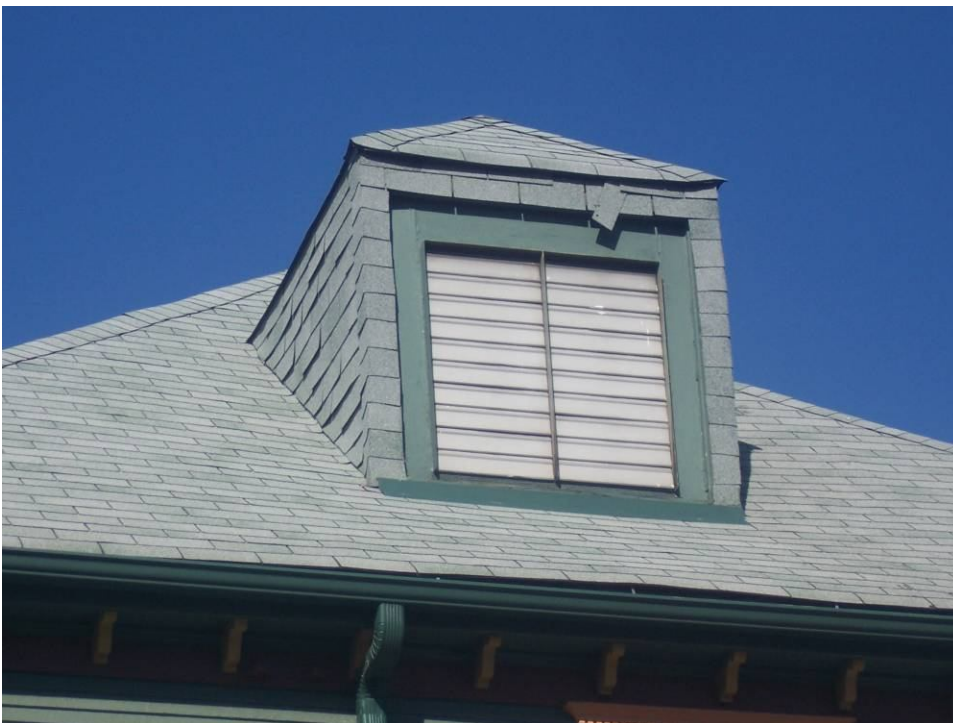
Asphalt shingles are not an appropriate siding material
