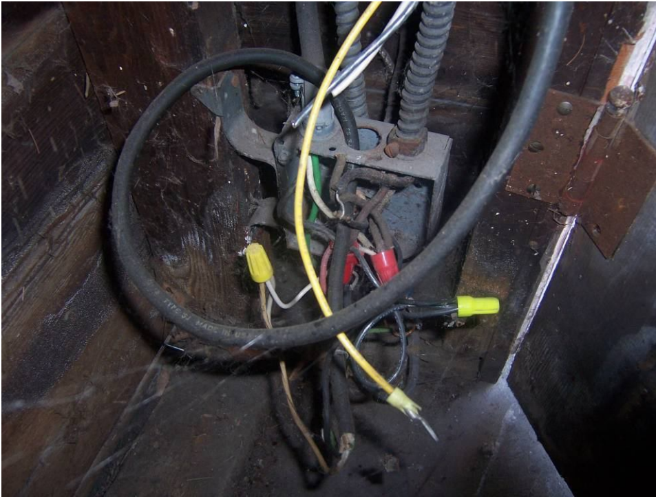
Garage wiring is unsafe - exposed wires
