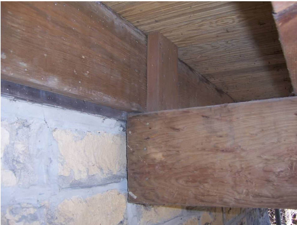
Rear deck is poorly supported at the house
