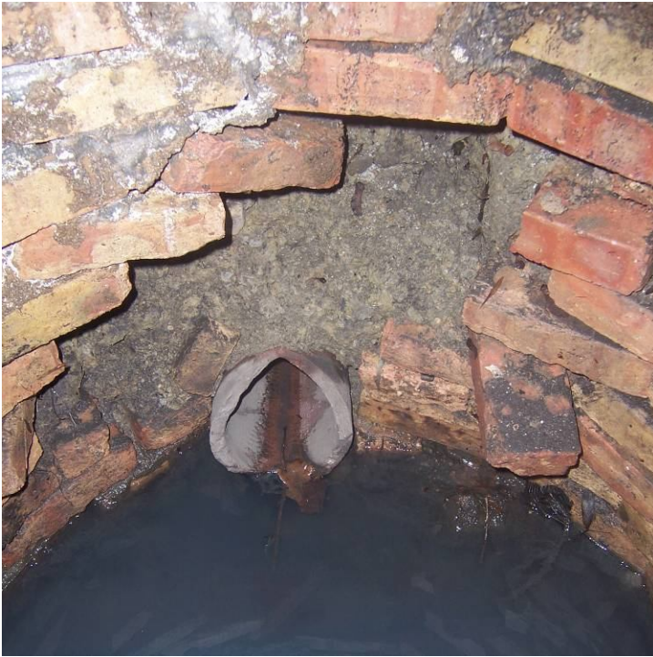
Bricks missing at grease trap – structure may collapse
