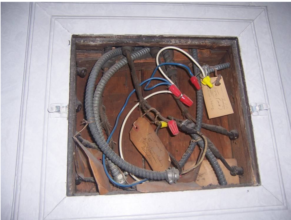
Electrical splices are not made inside an approved box
