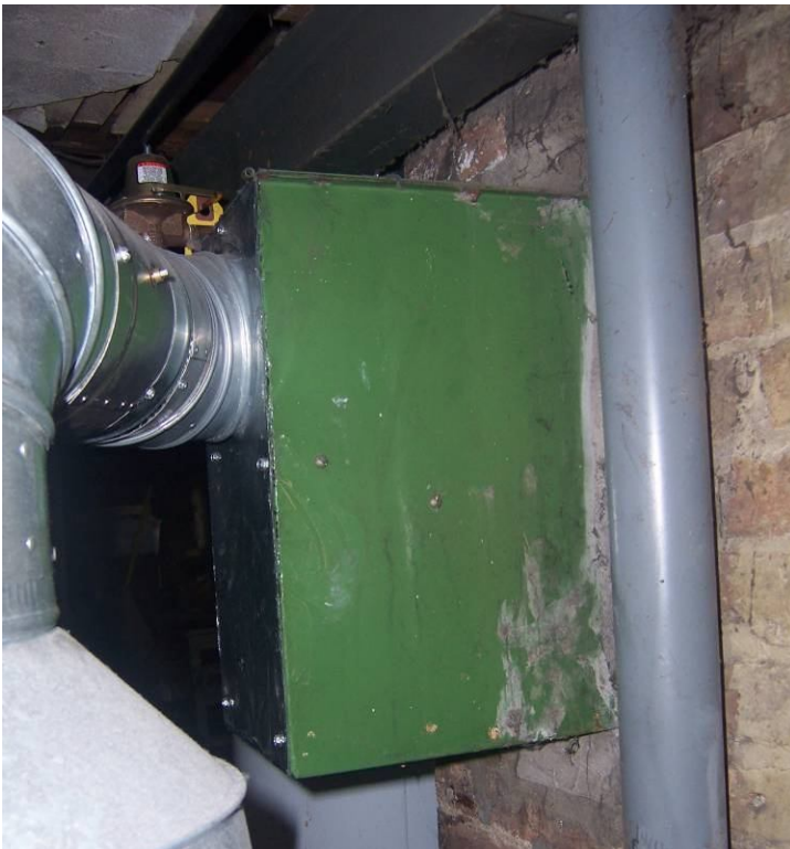
The boiler flue should enter directly into the chimney – the green box should be removed
