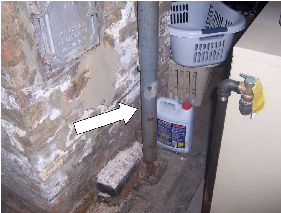
Support post in basement is not designed for permanent installation
