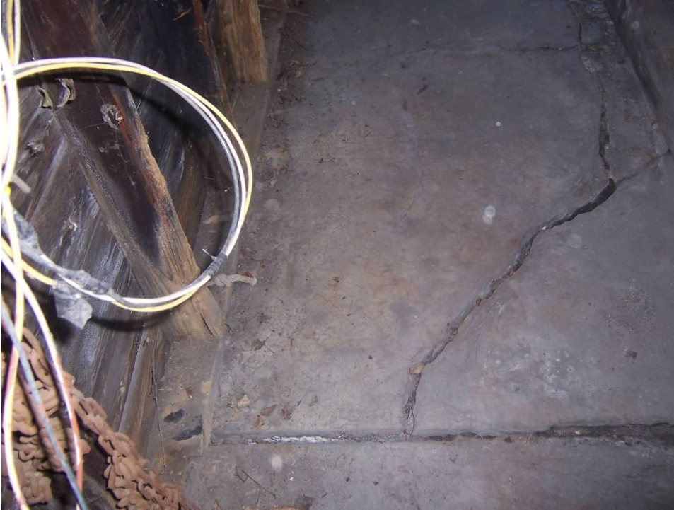
Garage slab and foundation have settled, and walls are not properly supported
