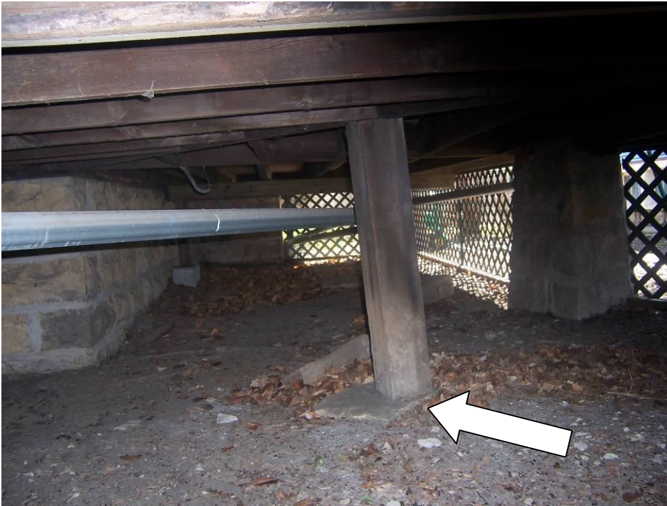
Front porch posts are poorly supported – they do not rest on a proper footing
