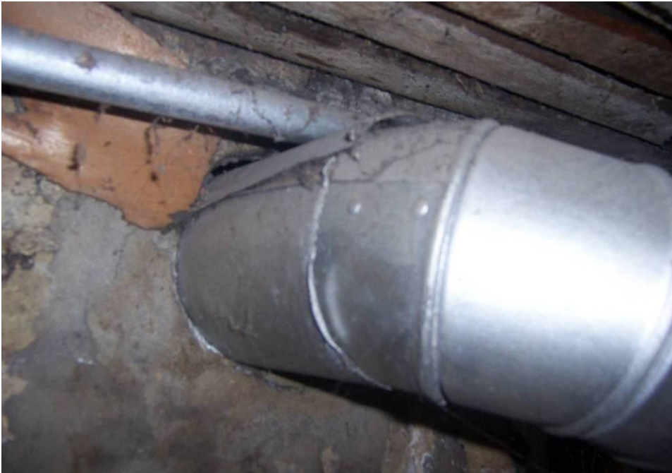
Water heater flue is poorly installed - unsafe
