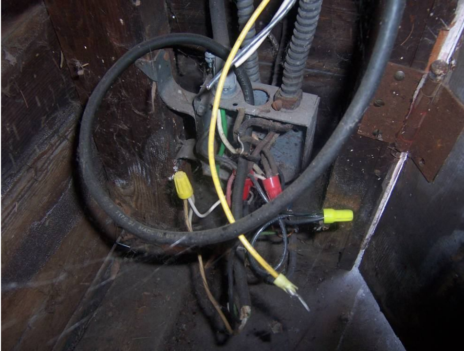
Garage wiring is unsafe - exposed wires
