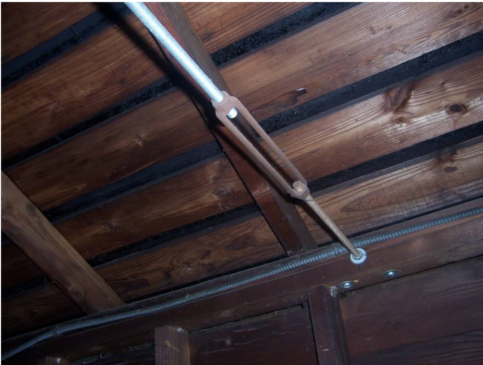
Steel rods have been added to support the garage walls – unsafe
